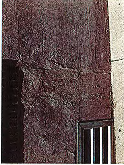
(Additional Spall Repair)
