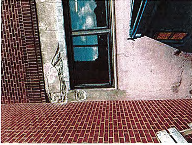
(Additional Spall Repair)
