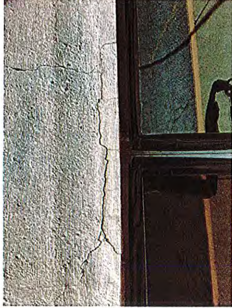
(Additional Spall Repair)
