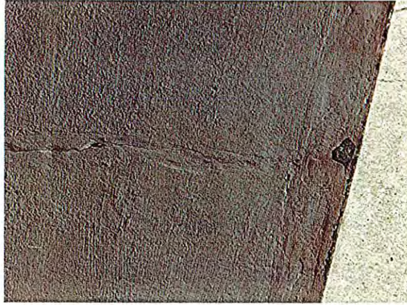
(Additional Spall Repair)
