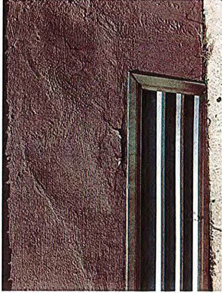
(Additional Spall Repair)
