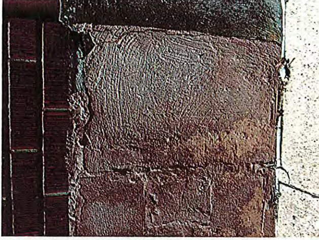
(Additional Spall Repair)
