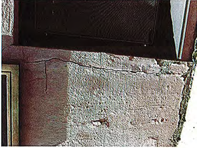
(Additional Spall Repair)
