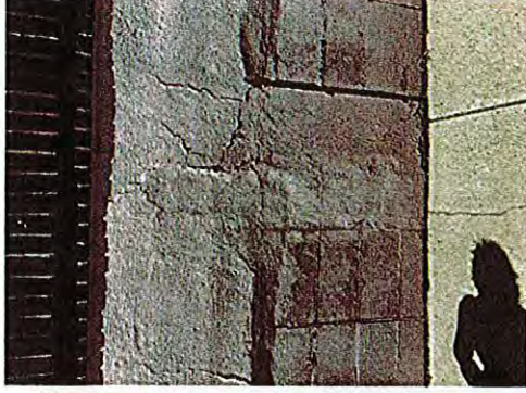
(Additional Spall Repair)
