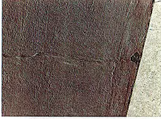
(Additional Spall Repair)
